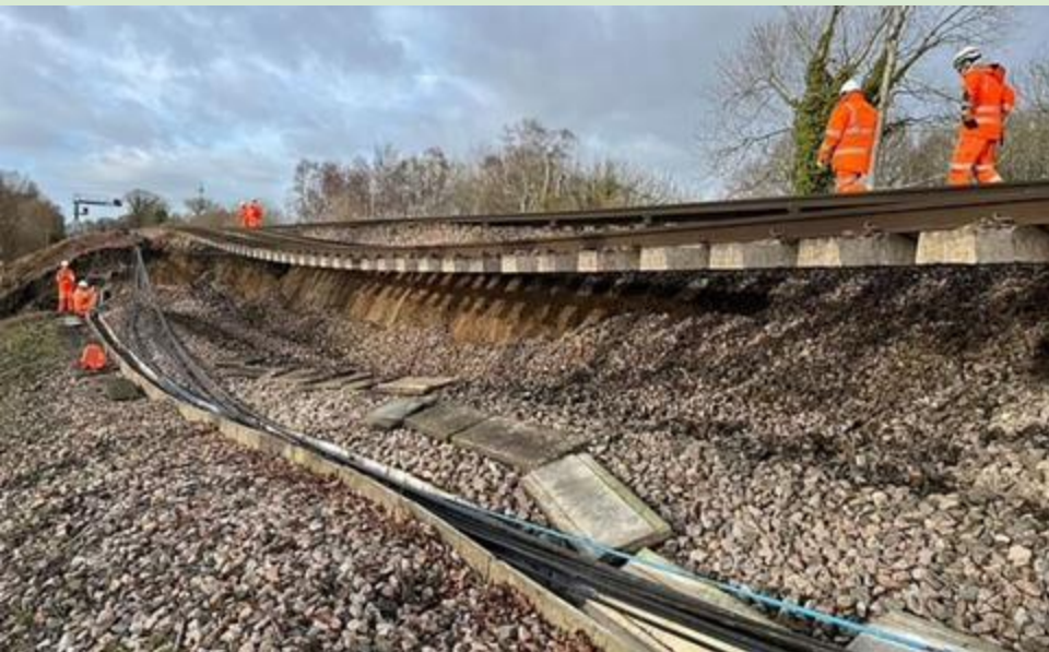
Hook Line collapse (Wok-Bas)
